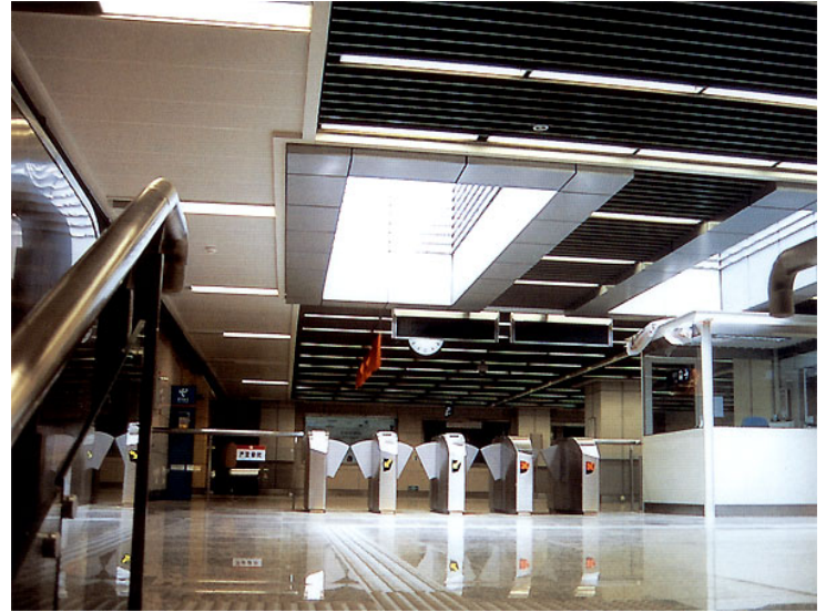
Figure 8. Subway Station Lighting
